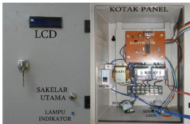
Figure 4. Overall Hardware View
