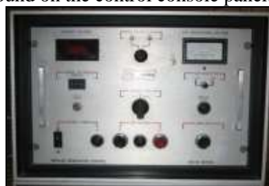
Figure 3. Front panel of the control console
